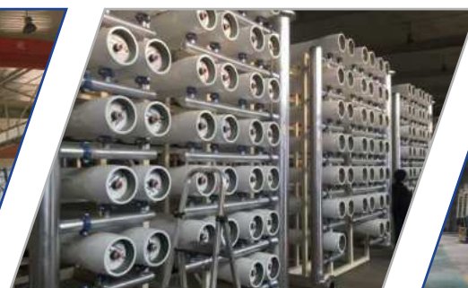
Qingdao wastewater reclamation project. Aug 2016
