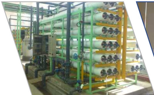
Gansu chemical plant water process engineering. May 2014
